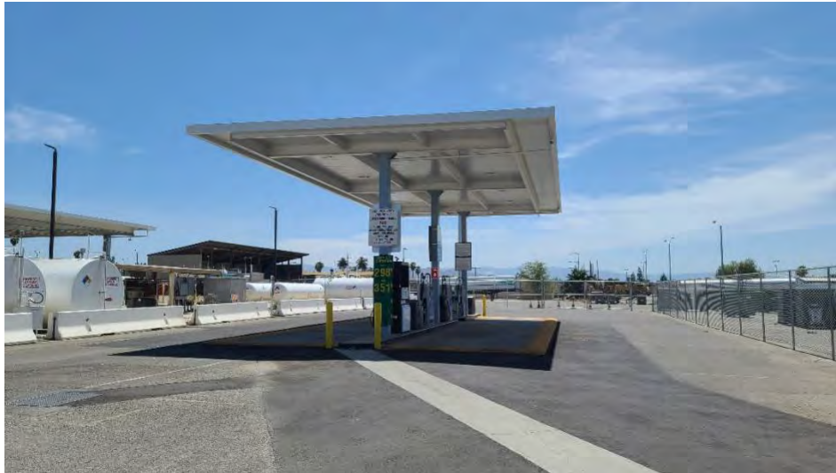
Satellite Fueling Island
