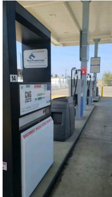
CNG Fuel Dispenser
