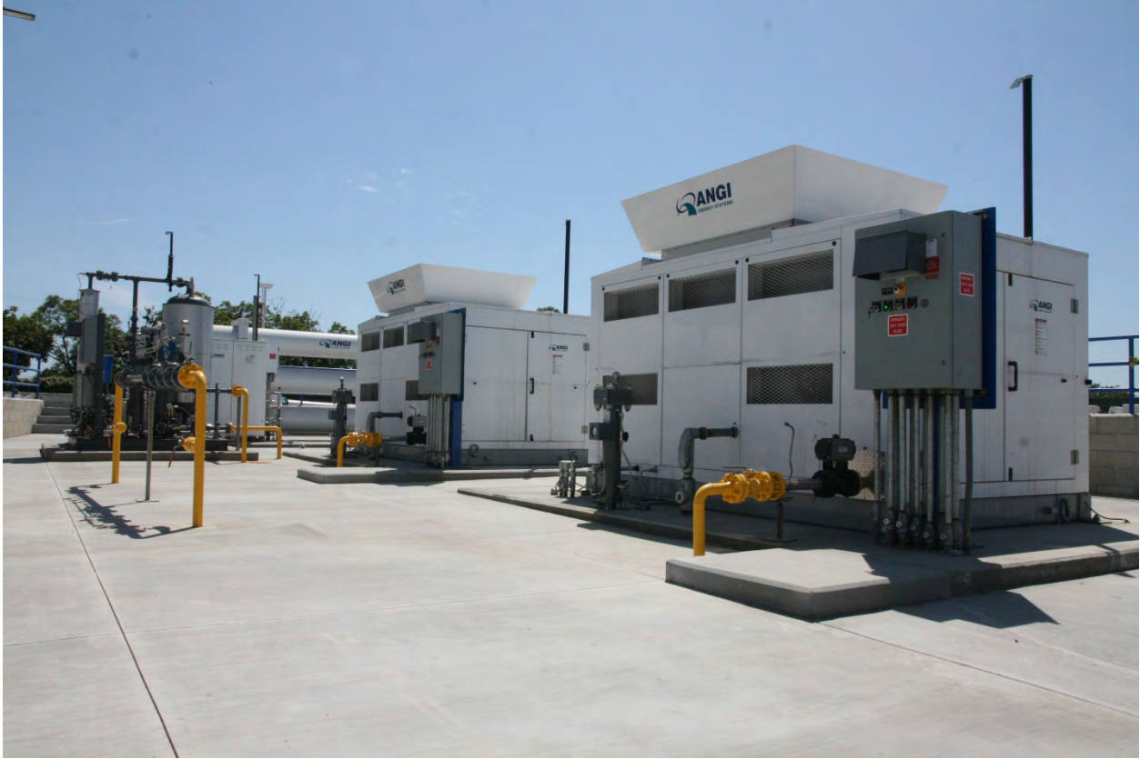
Figure 1: SoCalGas Compression, Dryer and Storage Facilities, Pico Rivera
