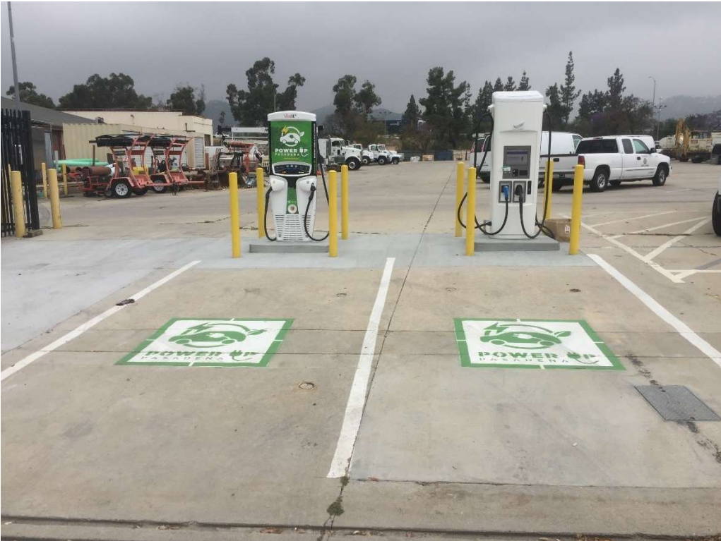
Two Fast Chargers at the City Maintenance Yards
