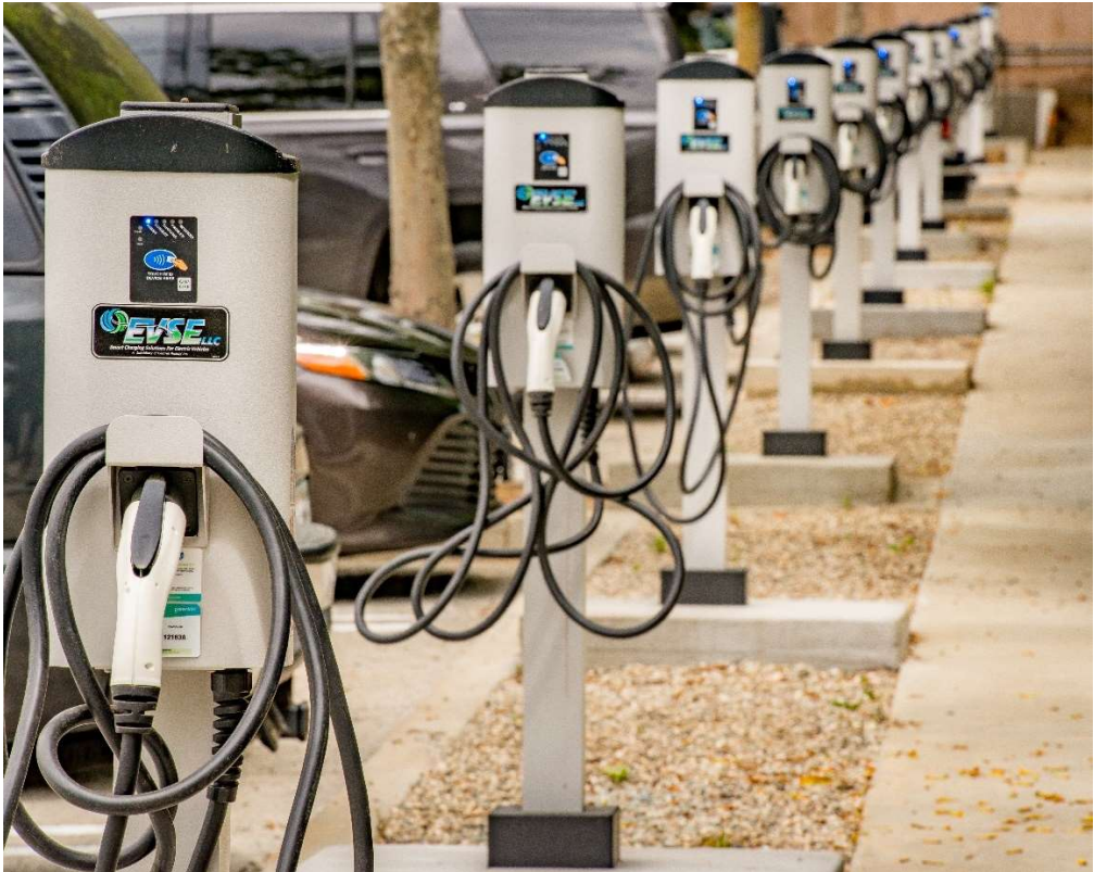
Fifty-five Level 2 chargers at the City Maintenance Yards
